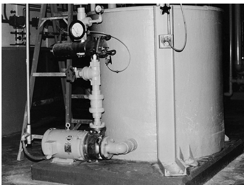
Reverse osmosis, Ósmosis invertida
